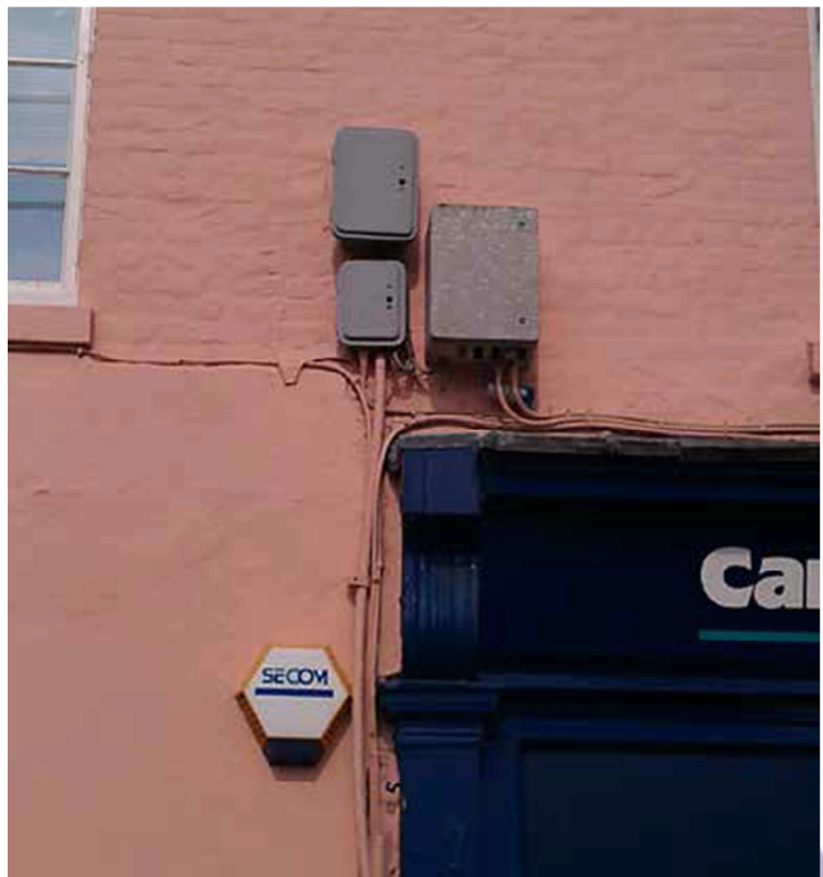
Alarm boxes should be as discreet as possible
